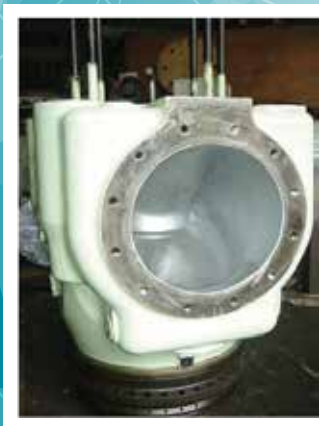
M/E EXHAUST VALVE HOUSING AFTER RECONDITIONED
